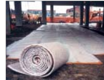
Finesse Gasflow - typical gas dispersal system installation
